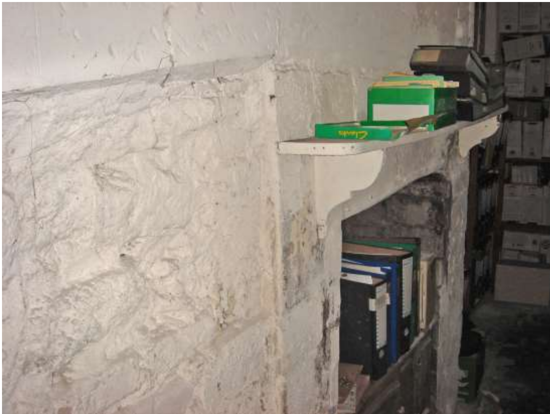
The blocked-in Tudor fireplace in the cellar of the Ralph Allen Town House, with a smaller fireplace inserted into the right side. See also page 54.
